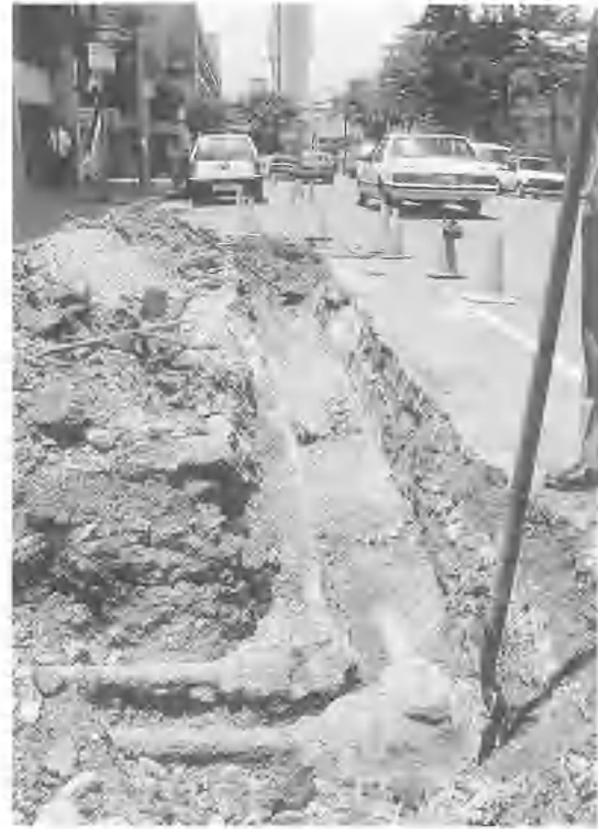
FIG. 7. The 1992 excavation of part of the mains in William Street in progress. The elbow joint boxes are seen in the foreground. The straight junction boxes are not yet exposed at the further end of the trench. The tall building in the background is the modern (1980s) extension to the Parliamentary Buildings. The sharply pitched roof of part of the 1892 extensions is just visible above the tree-line.
